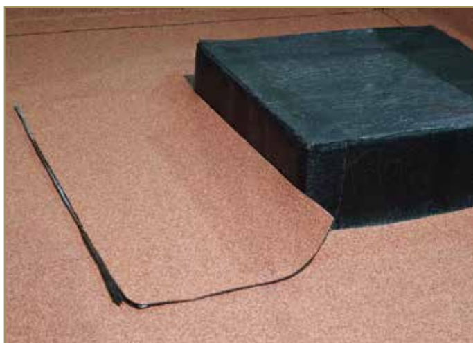
Figure 9.52: Preparing the vertical up-turn of the second waterproof layer with slate chipping finish
