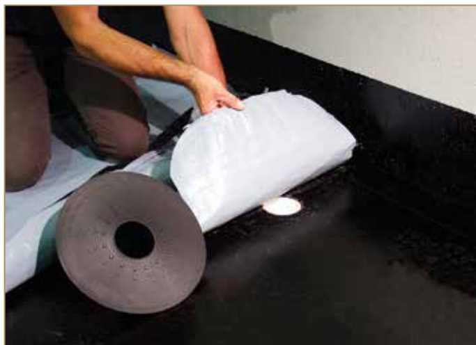
Figure 9.69: Preparing the membrane to place under the outlet flange for vapour barrier 50x50 cm
